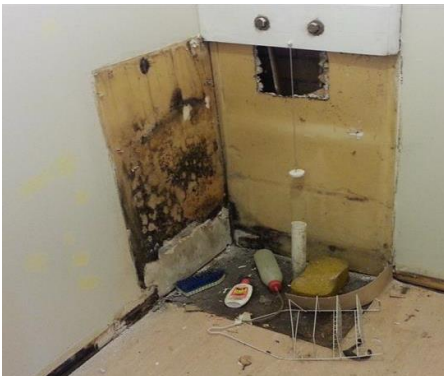
Plumbing pipe leaks
