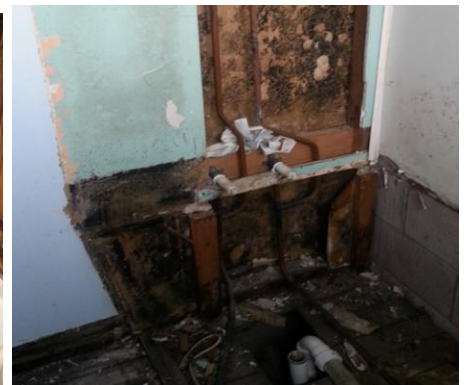
Mould can often be hidden behind wall linings
